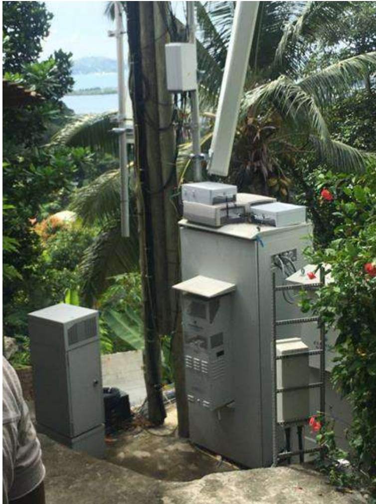
Figure 42 - Mt. Buxton: base station infrastructure at MP1
