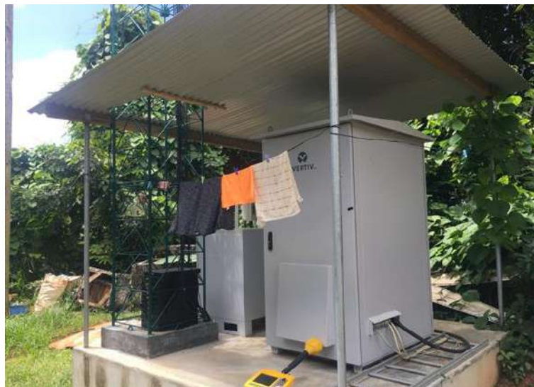
Figure 37 - Ma Constance: base station infrastructure
