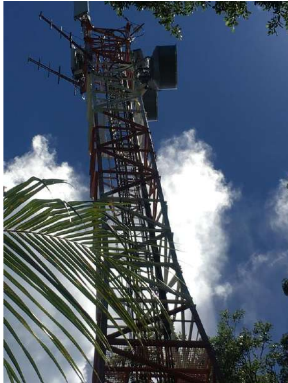
Figure 115 – Port Cabris: identification of base station (CWS)
