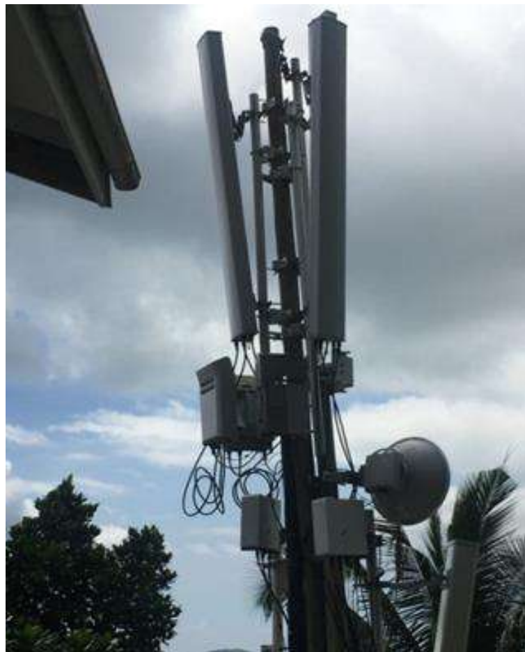
Figure 41 - Mt. Buxton: proximity of base station to MP1
