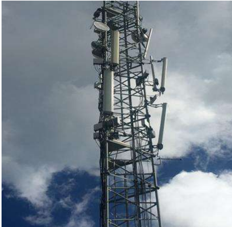
Figure 72 – Hermitage (SBC): identification of base station
