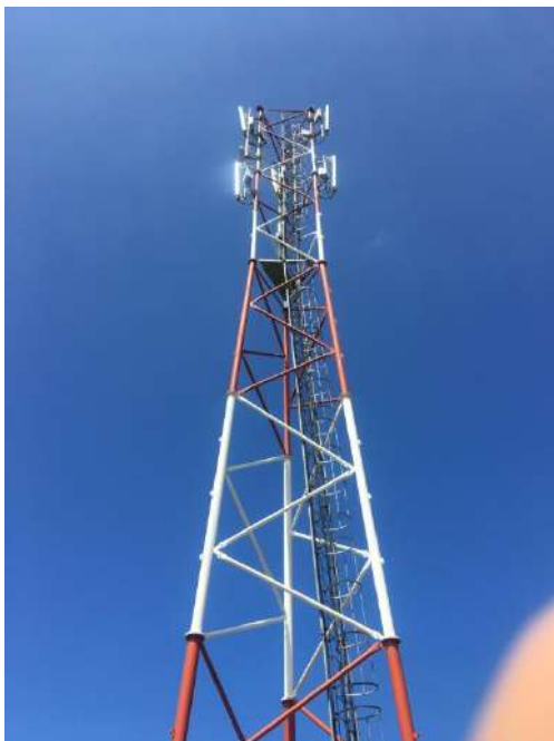
Figure 105 – Port Launay: identification of base station
