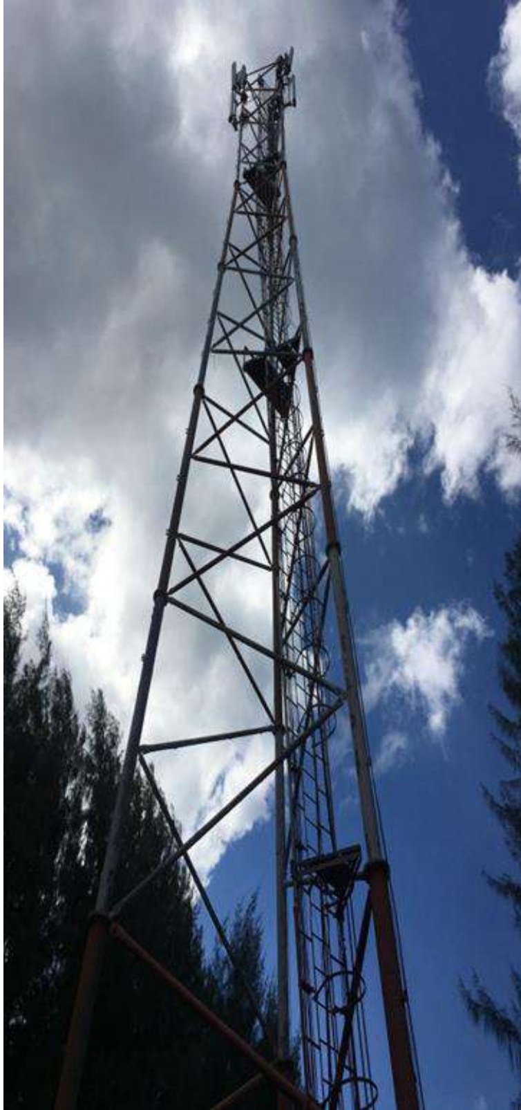
Figure 29 - Perseverance: viewed from MP2 location
