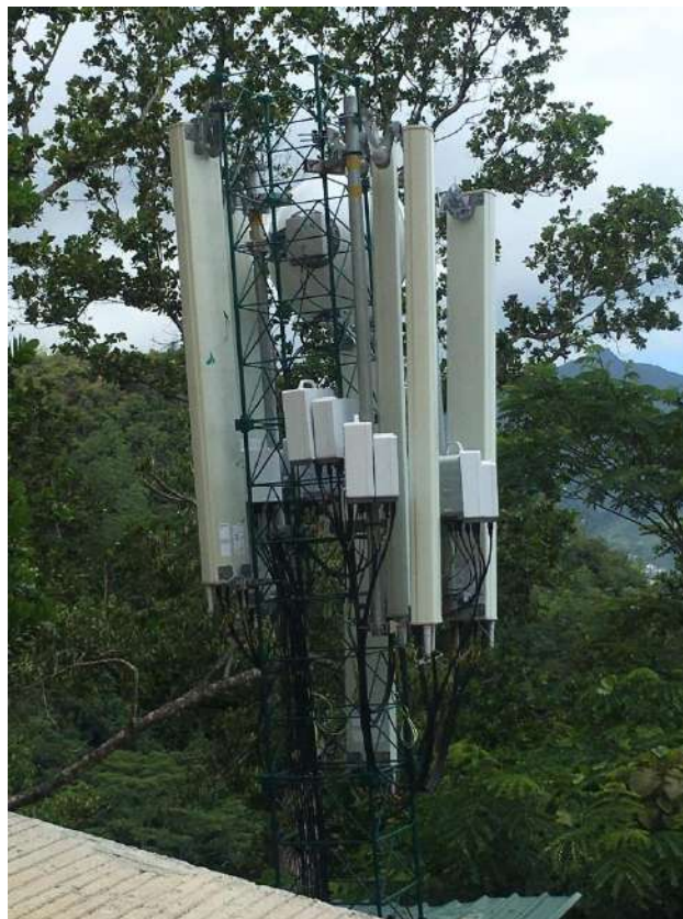
Figure 18 – Sorento: view of base station
