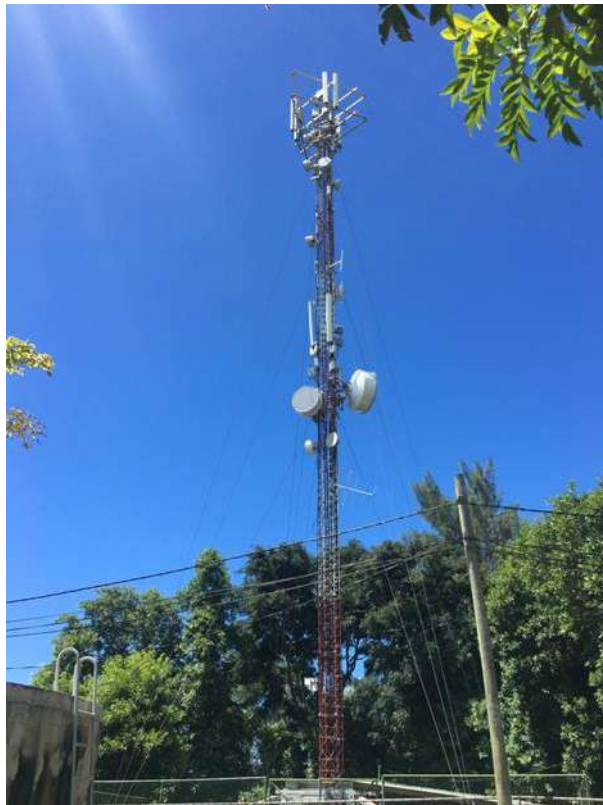
Figure 116 – Port Cabris: identification of base station (Airtel)
